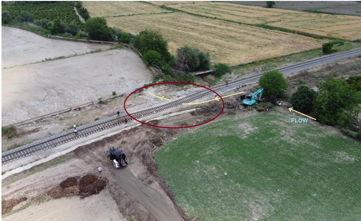
Figure 8. During the flood, the soil under the tracks was washed away and the railway line collapsed.
