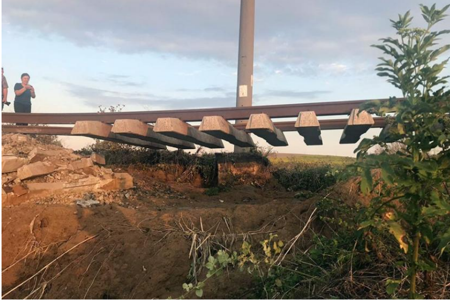
Figure 6. The ballast and foundation material on the culverts washed away by flowing water over the infrastructure
